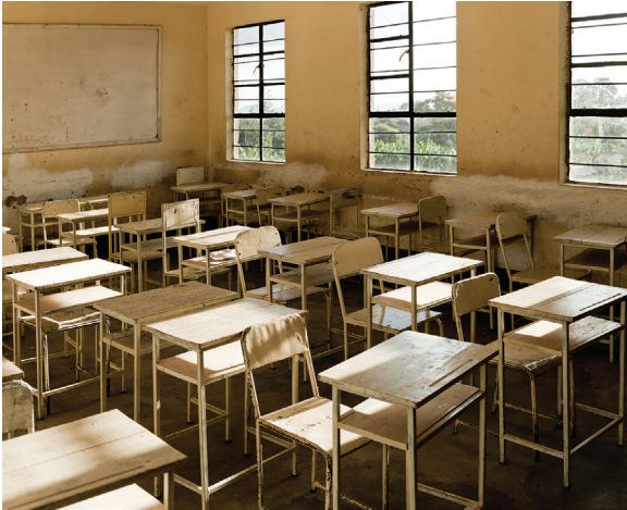
Dilapidated schools have to spend funds for repairs that could otherwise be used to purchase instructional materials or pay higher salaries to more qualified teachers.
